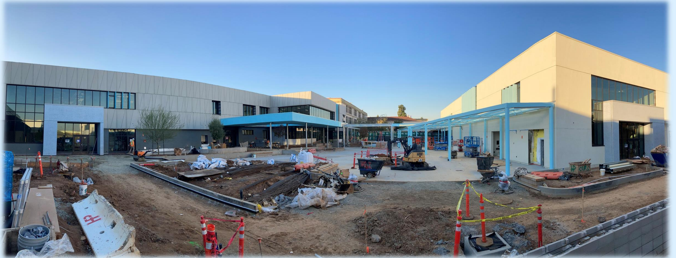
In Construction: New Administration/Classroom Building (left) and New Food Service Building (right)
