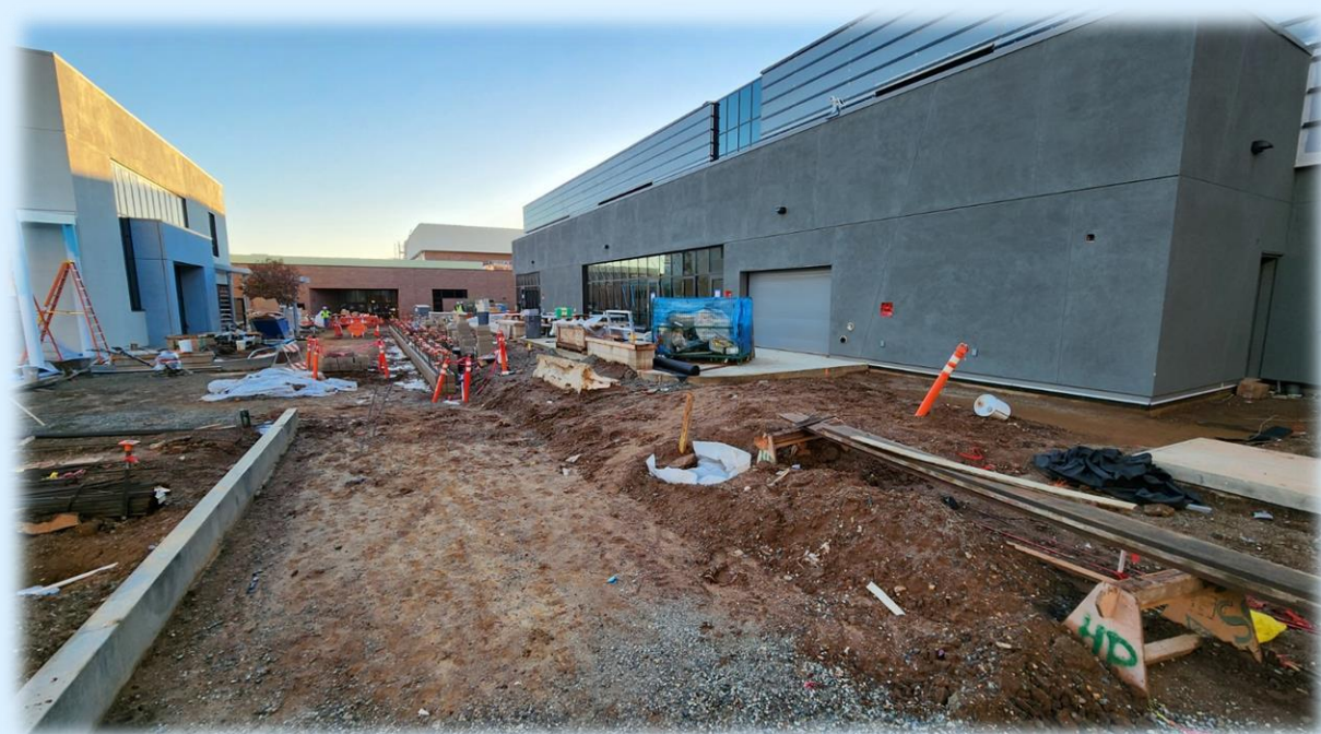
In Construction: New Classroom Building (right) and New Food Service Building (left)
