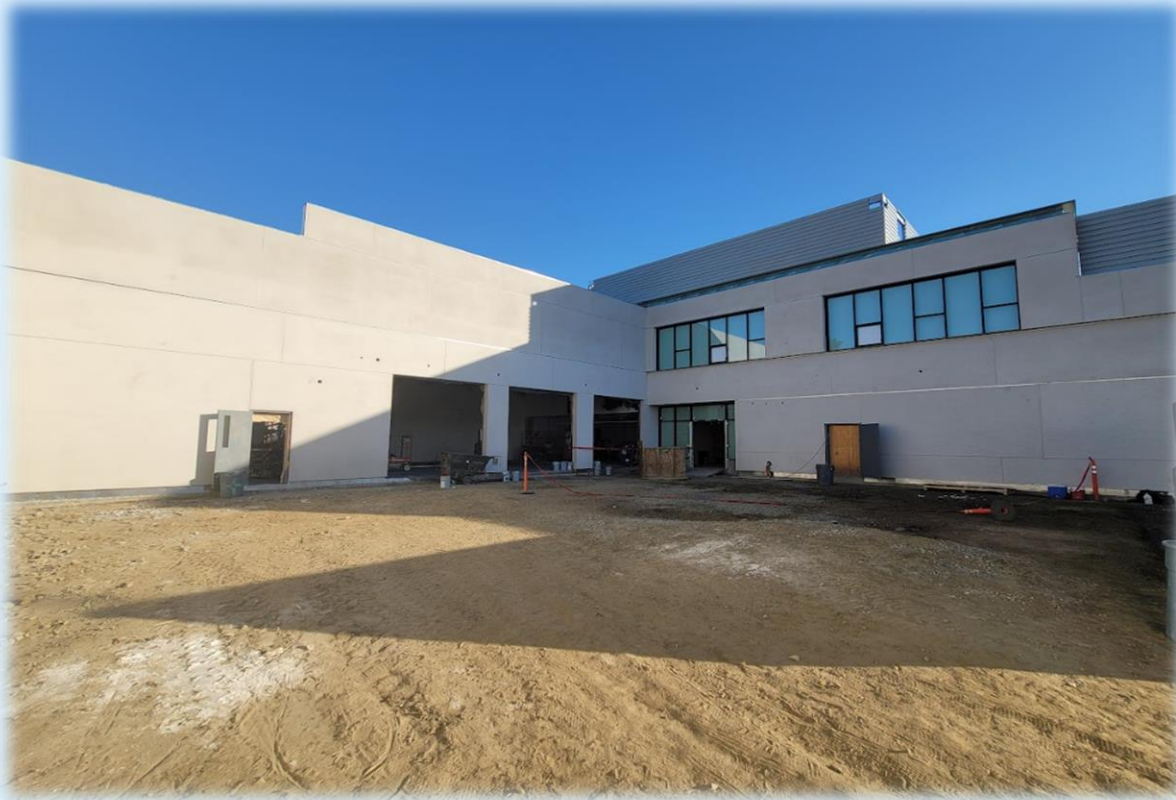
In Construction: Exterior of New 2-Story Classroom Building, Robotics, and Auto Shop
